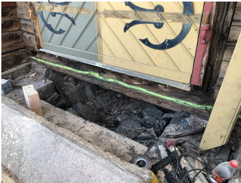
Skador under port
